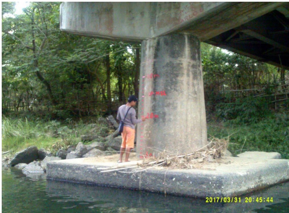
Figure 45. Water-level markings on the pier of Lumang Bayan Bridge
